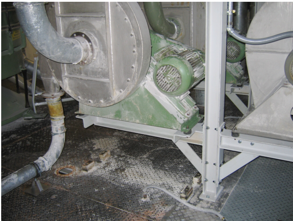
Illustration: Fans installed so that vibration is not transmitted to the bearing plate
